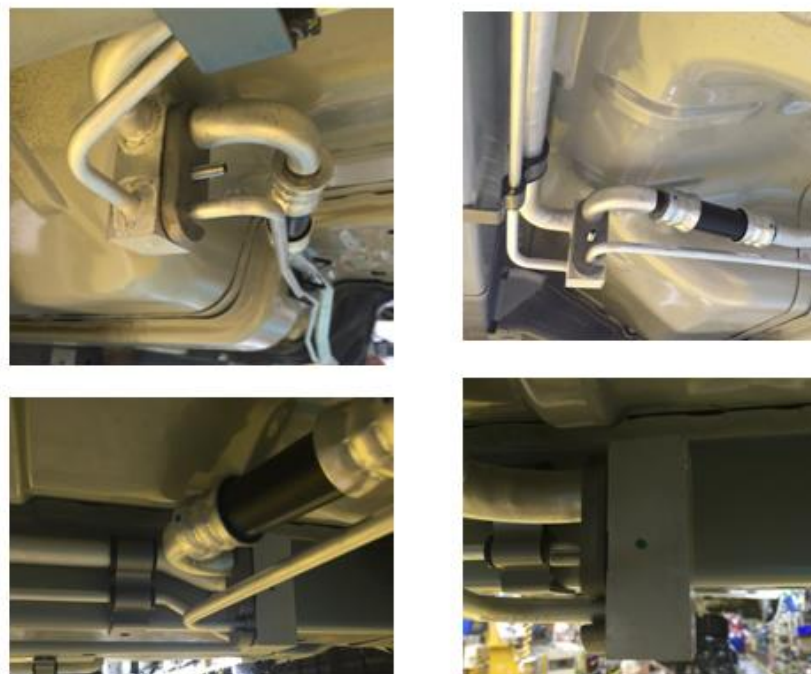
Front auxiliary AC lines Off-line trial after design improvement
