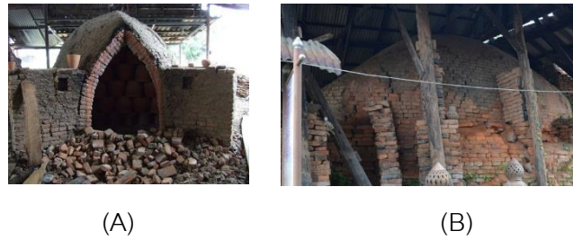
Figure 2: the Front Side (A) and the Curved Roof the Mon Kiln (B)
